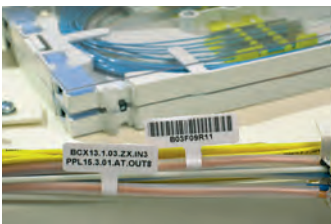
Fibre optic cable markers
